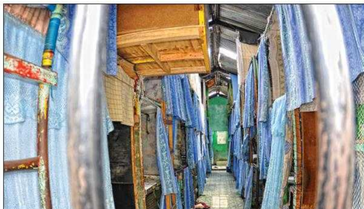
This view into a cell at Comayagua, looking down the center aisle toward the bathrooms at the rear, shows the extent of the cloth, wood, and other combustible materials used by inmates to customize their bunk areas. ATF investigators estimated that each module at the time of the fire included approximately 6,288 square feet (584 square meters) of draped cloth and 538 cubic feet (15.2 cubic meters) of mattress padding. Photo: Jaime A. Moncada.
