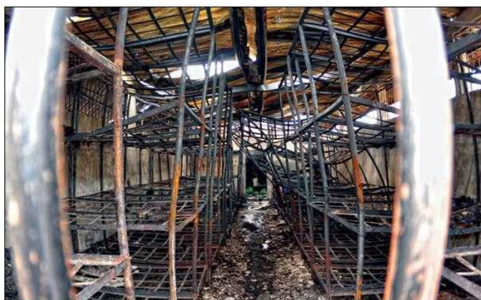
The abundance of fuels in the modules resulted in an intense fire that grew rapidly. The ATF report found that, by the time it was extinguished by fire crews, the fire had consumed almost every speck of combustible material. Photo: Jaime A. Moncada.
